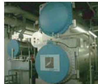
Heat pump for utilizing sewage water heat
