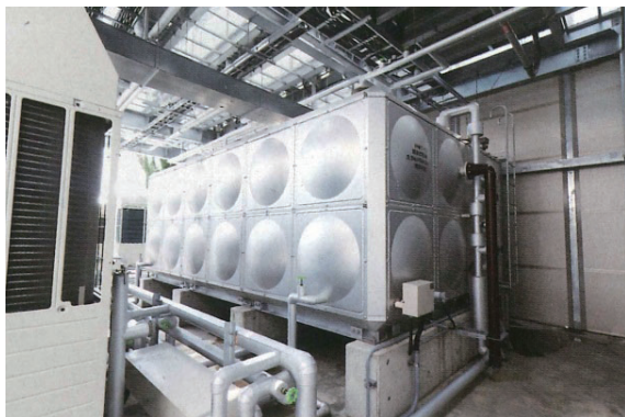
EcoCute Hot Water Tank
