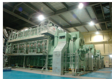
Inside electric generator room at Nihon Techno
