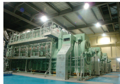
Inside electric generator room at Nihon Techno
