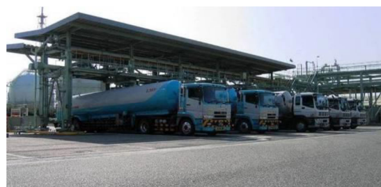
LNG tank lorry shipping facility
