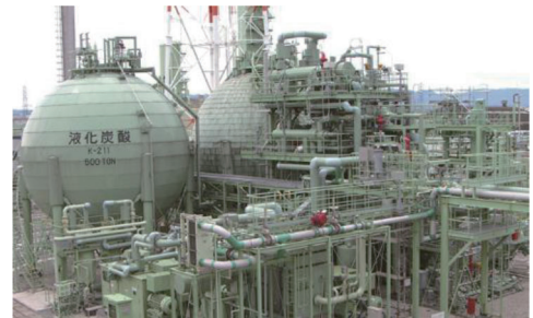
CO 2 liquefaction facility
