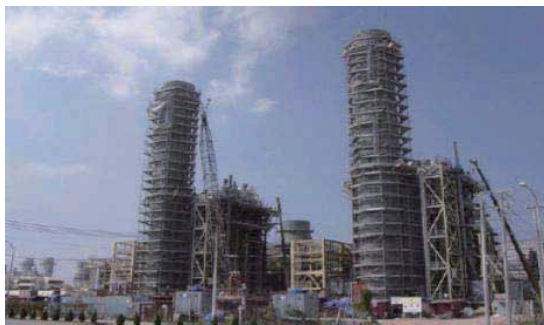
Heat Recovery Steam Generator in the Phu-My 2-2
