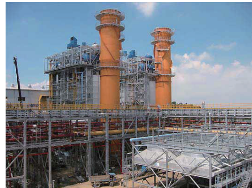
Chang –Bin Power Plant (Taiwan)
