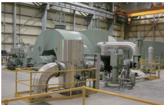
Geothermal steam turbine and generator
