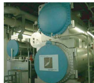
Heat pump for utilizing sewage water heat
