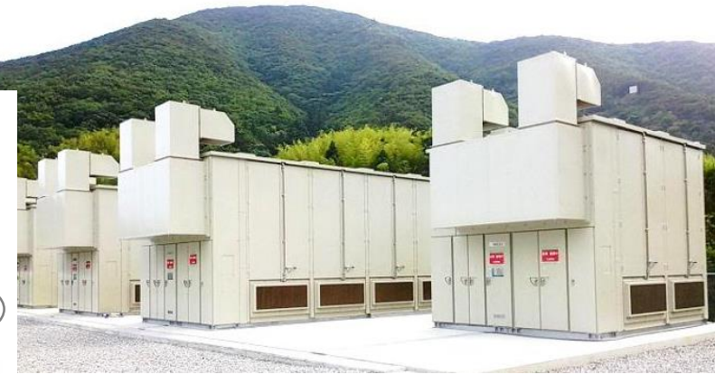
4.2MW of NAS ® Battery System
