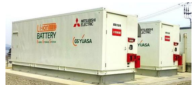
2MW of LiB System
