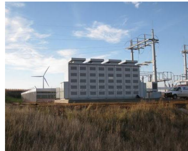
NAS Battery system for Xcel Energy (1MW, COD 2008)
