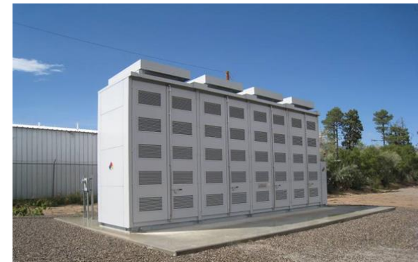
NAS Battery system for Los Alamos (1MW, COD 2013)
